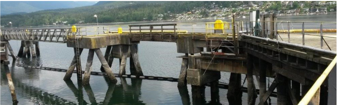
Location of DAS Sonar. Note the angle of the pilings as they enter the water.
